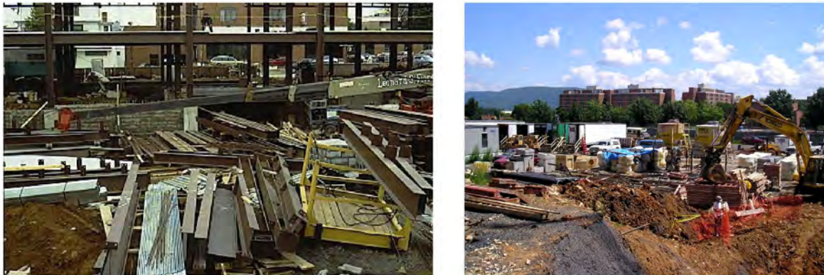
FIGURE 3.1 Examples of poorly managed job sites. SOURCE: Thomas (2008).
